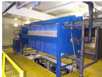
IWWS Filter Press dewateres sludge
