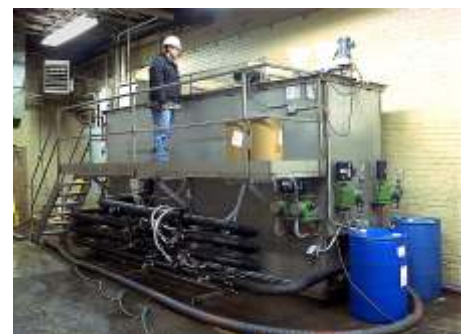
200 GPM Continuous Metals Removal System
